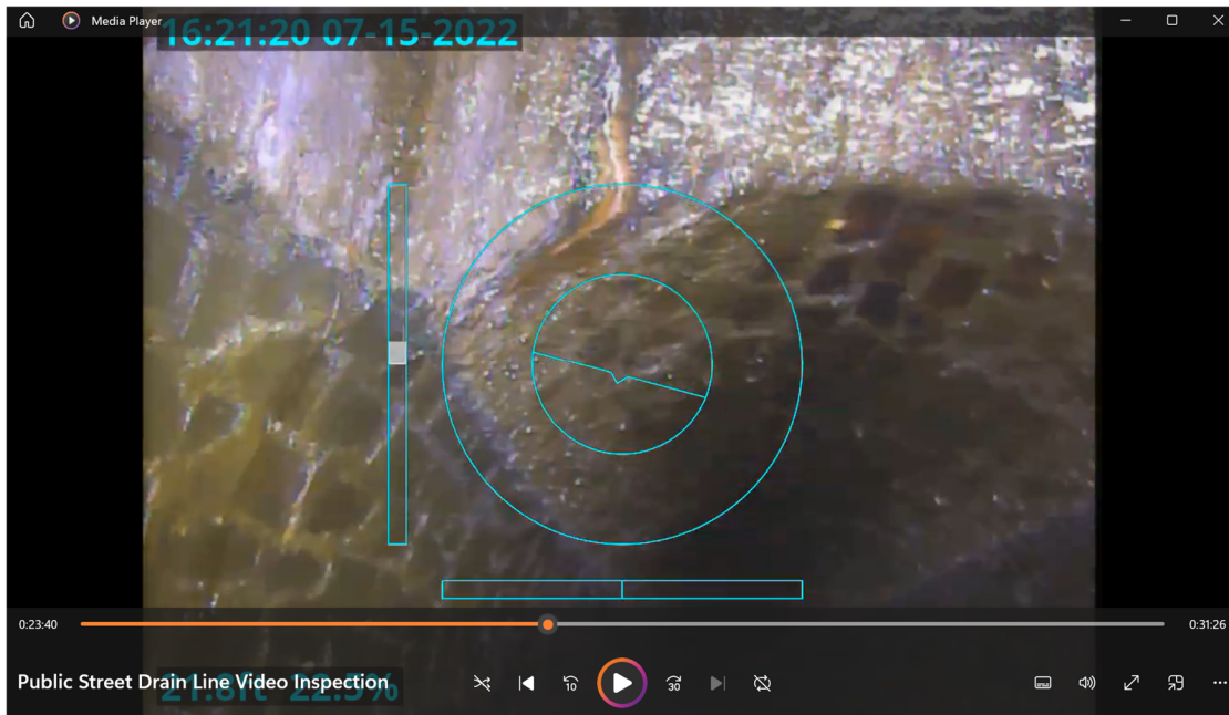
Photo 1: Active water infiltration observed in video
