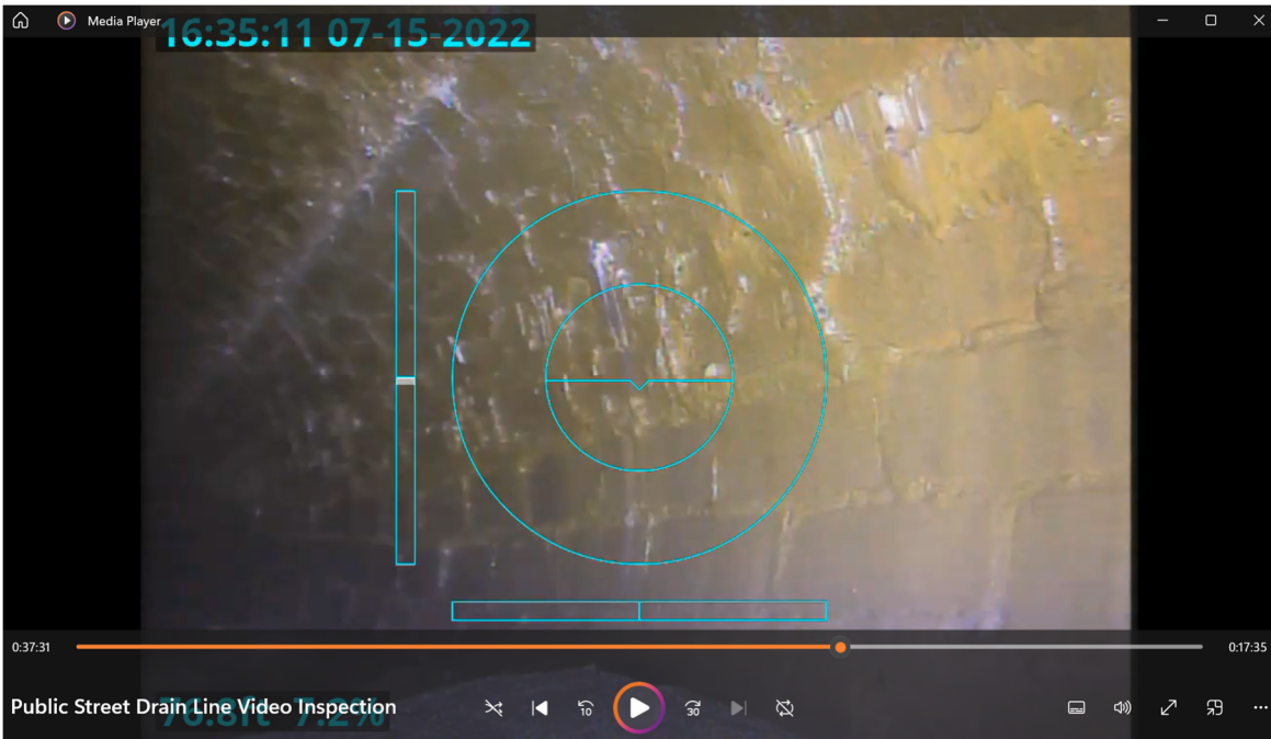
Photo 8: Calcium staining indicating long-term water leakage
