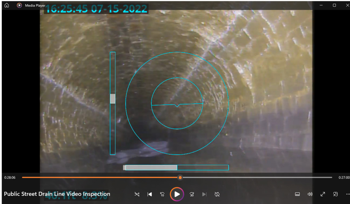
Photo 5: Calcium staining indicating long-term water leakage
