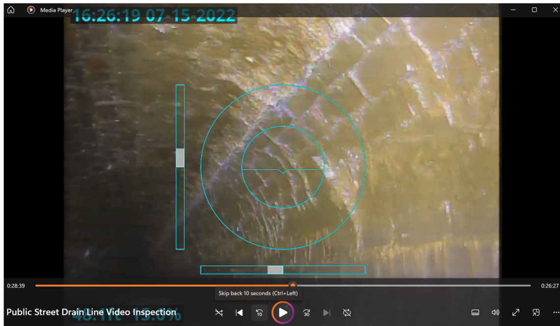
Photo 6: Calcium staining indicating long-term water leakage
