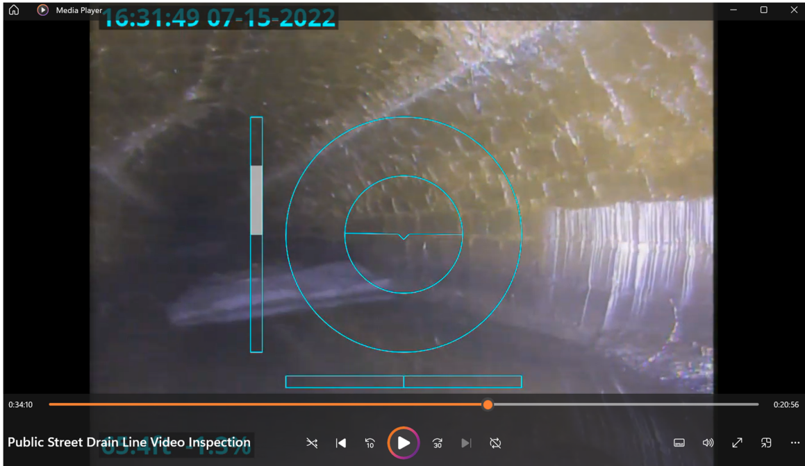
Photo 7: Calcium staining indicating long-term water leakage
