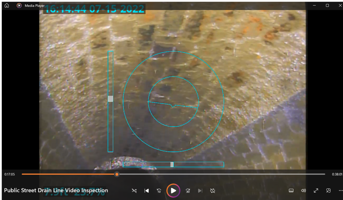
Photo 3: Calcium staining indicating long-term water leakage
