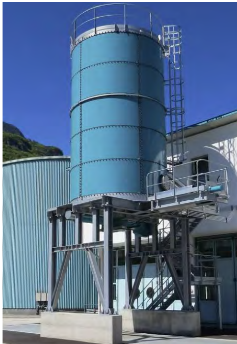
Figure 6 Example of Dried Feedstock Silos
