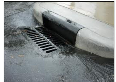
Stormwater runoff entering a storm drain
