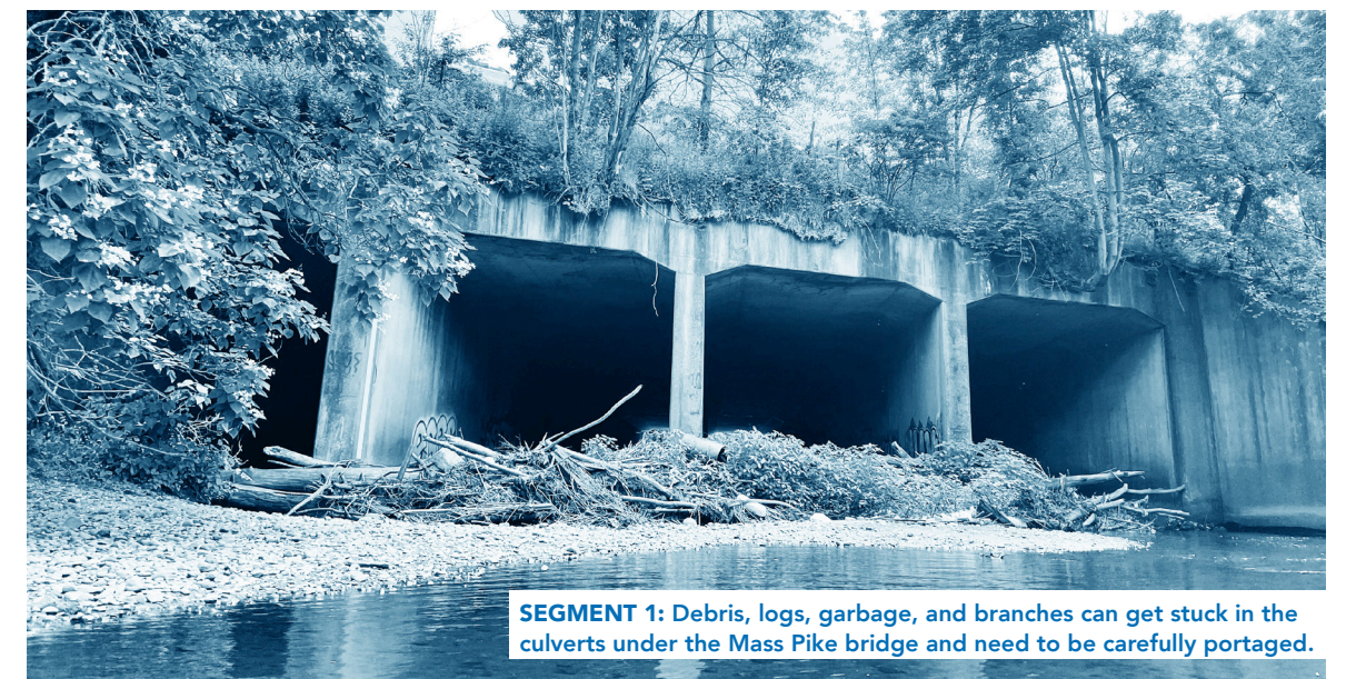
SEGMENT 1: Debris, logs, garbage, and branches can get stuck in the culverts under the Mass Pike bridge and need to be carefully portaged.
