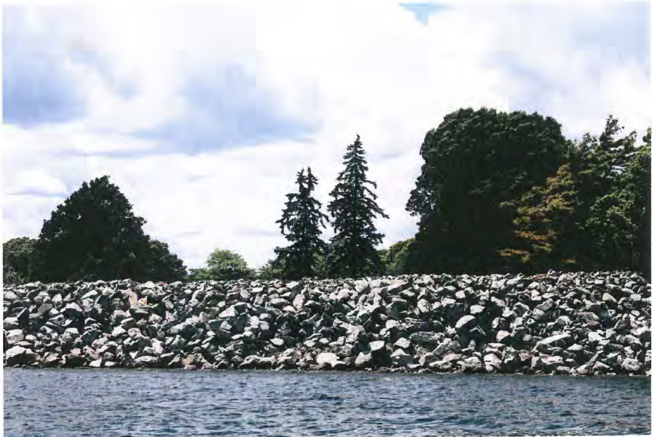
Close-up of illegal wall (Northern end) at High Tide of 4.1 ft on June 12, 2024. Note lack of passable shoreline indicating fill below Mean High Water.
