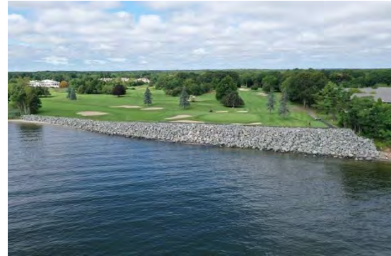
Figure 1 -QCC Illegal Seawall
